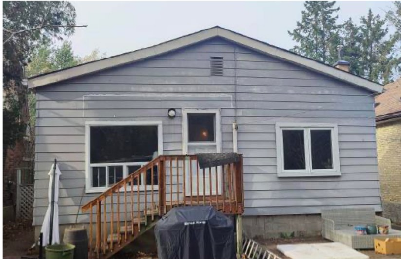
Figure 2: South (rear) elevation of the house showing the 1967 addition proposed for removal
